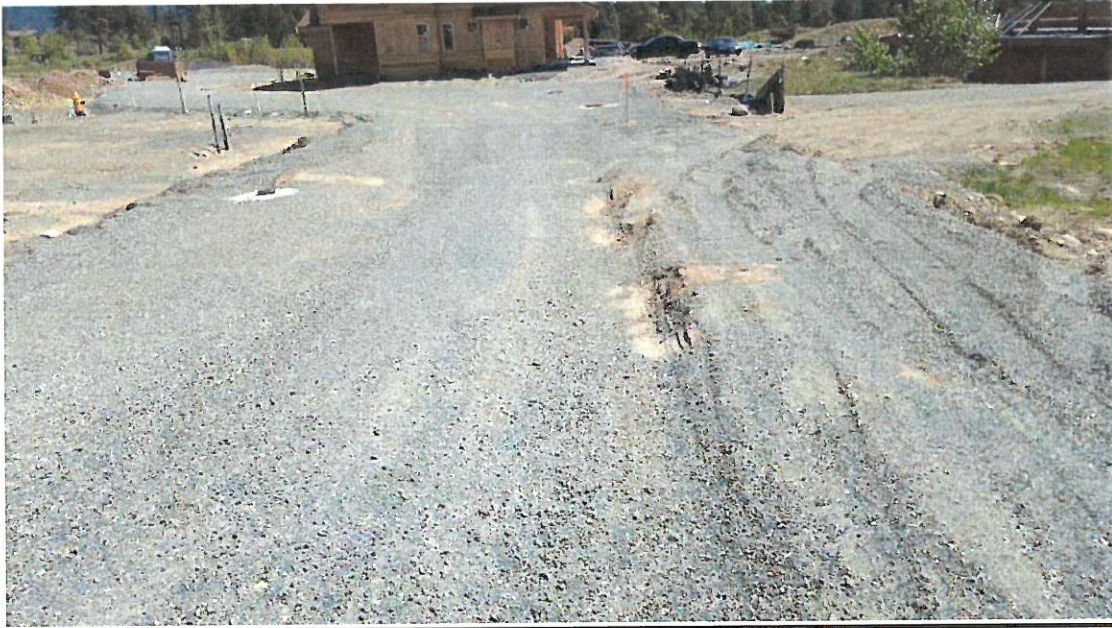
West entrance showing rutted area
